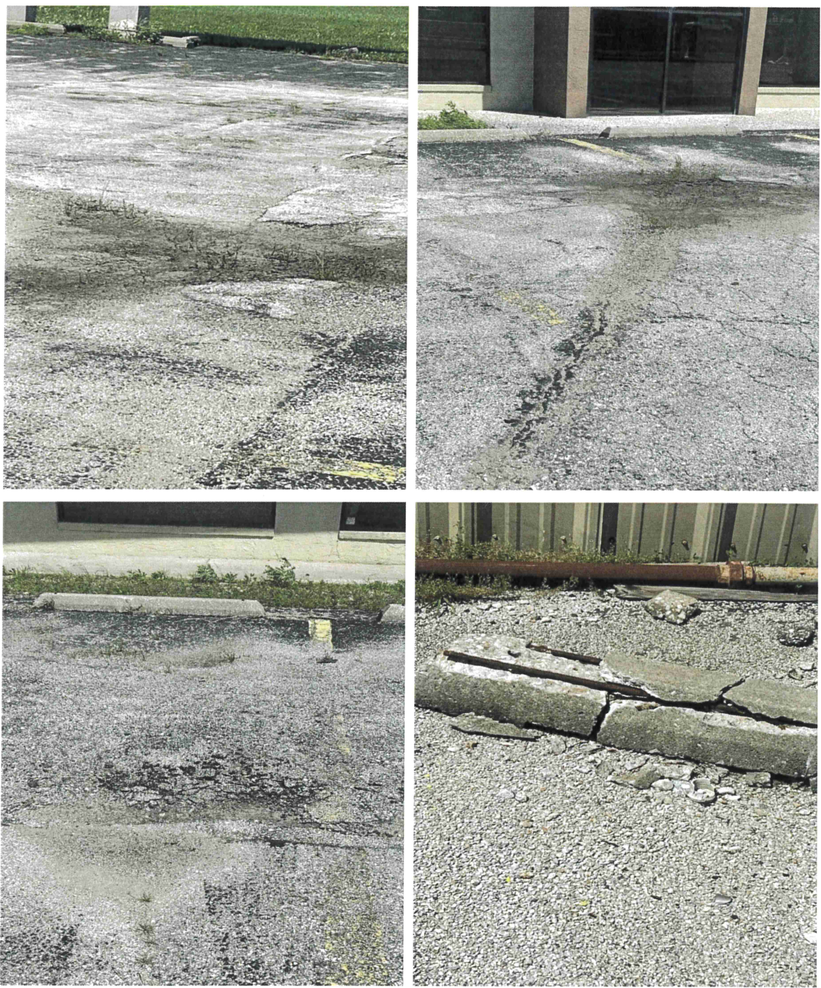
Figure 7: Deteriorated Parking Improvements
